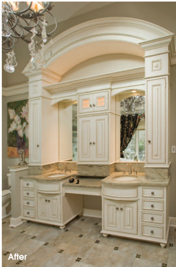
Although removing the dividing wall between the two rooms of the bathroom eliminated the sense of disconnection, it created an uneasy vastness. This was tamed through innovative use of color, accent moldings and cabinetry.
